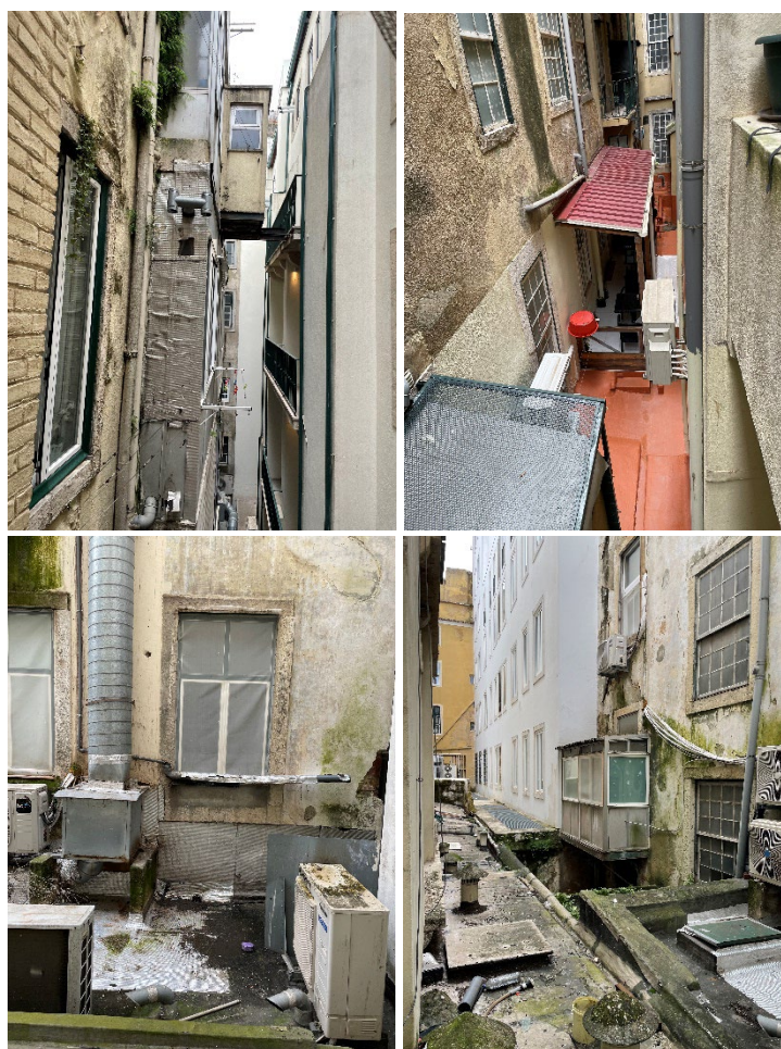
Figure 4. Some views of hallways with disruptive interventions and construction anomalies
