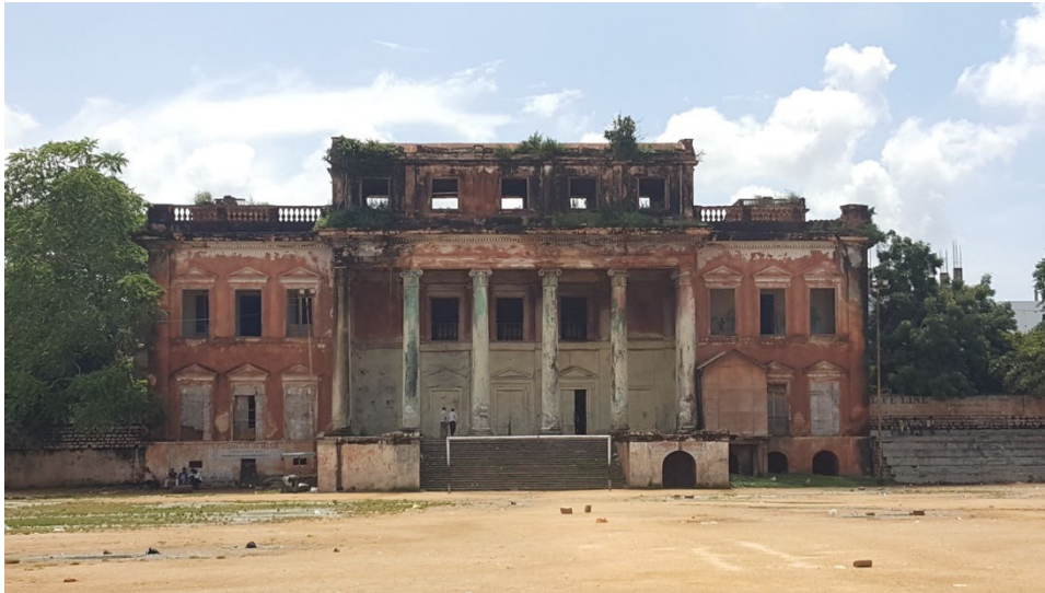
Figure 5. Baradari of Nawab Khursheed Jah Bahadur, Hyderabad, Photo Documentation by Ketham's Atelier Architects and Thinking Hand NGO Team.
