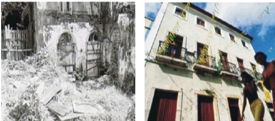
Figure 6. The property, which had become completely ruined after a fire followed by a collapse, was transformed into the first ten residential units of the program, with two shops on the ground floor. Source: Andres, 2006
