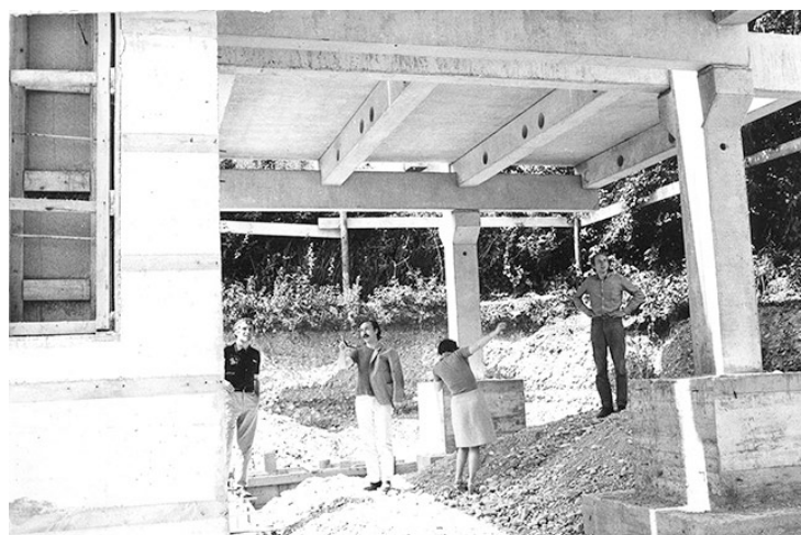
Figure 1. Doris and Ralph Thut with Otto Steidle (on the left) and Jen Freiberg on the building site of the Genterstraße housing project. Thut Archive.
