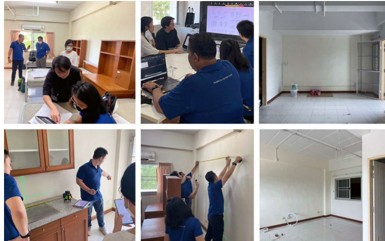
Figure 6. The renovation process of the two units: a single room with a kitchen and a twin room
