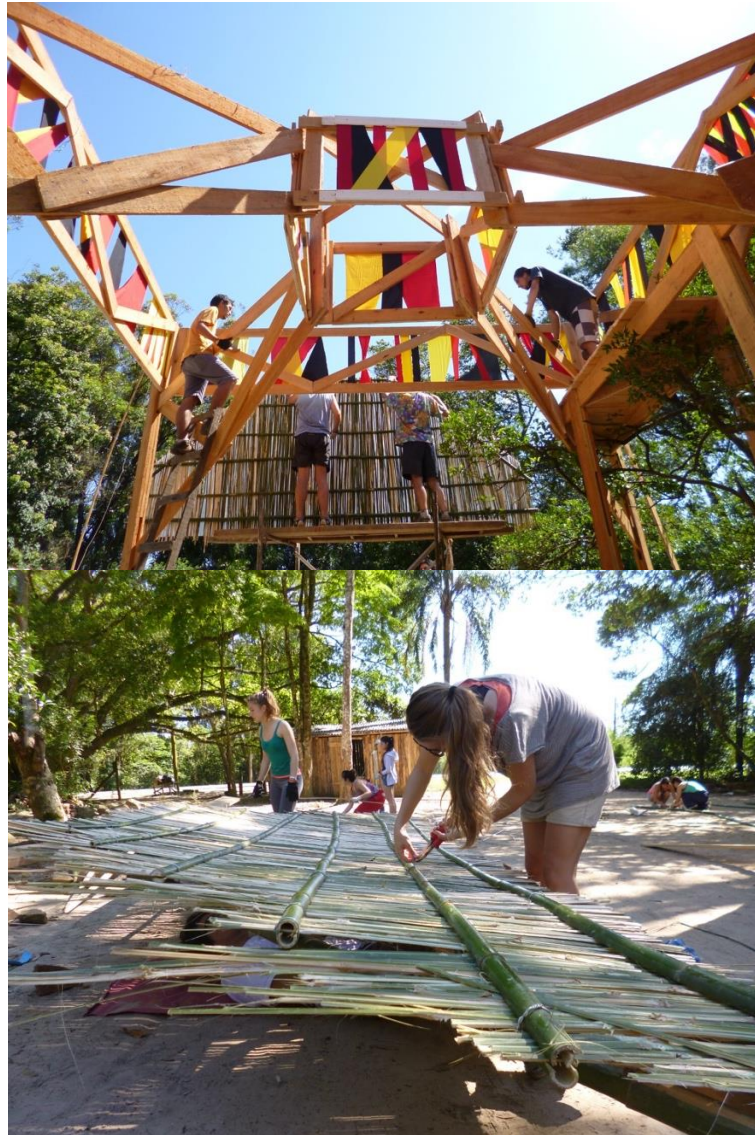
Figure 4. Wooden structure, trusses, and construction of the roof trapezoidal panels, by Oscar Andrade Castro.
