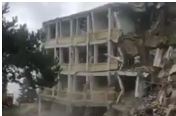
Figure 50. The demolition moment of the Ballıdağ sanatorium building captured from a video Source: Kastamonu Açık Söz newspaper, 6 September 2021
