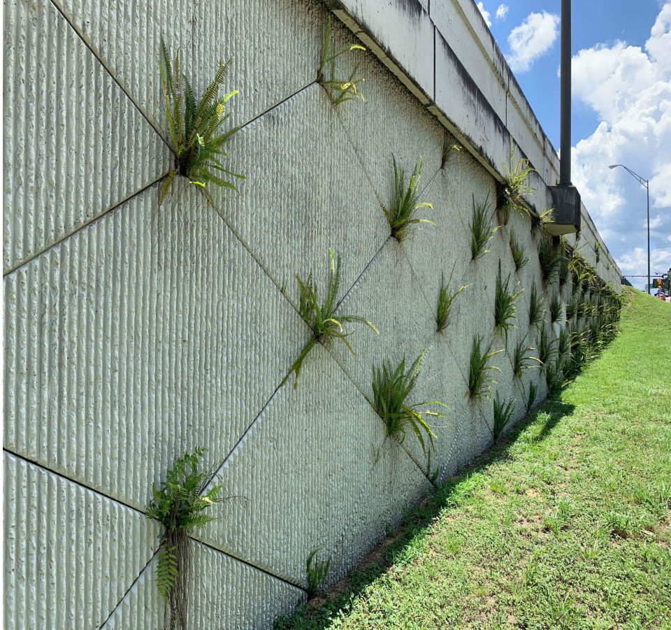
Figure 4. Ferns growing in the gaps of the MSE walls of an overpass in Tallahassee, FL. Courtesy of Apex Architecture.
