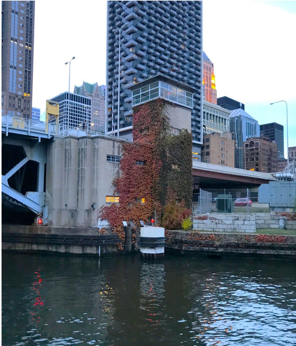
Figure 3. Vines growing on abutment of a bridge in Chicago, IL. Courtesy of Apexx Architecture.
