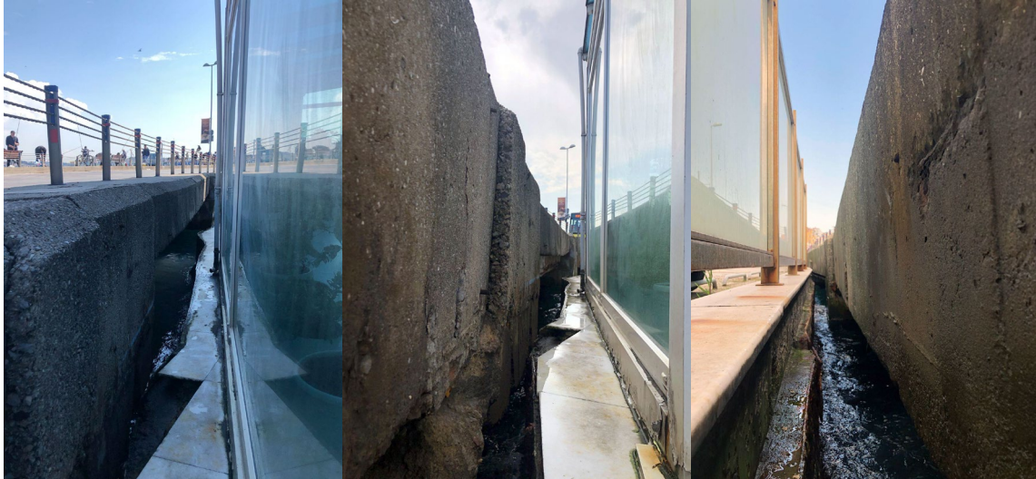
Figure 7-8-9. The threat the road poses to the structure. Source: Authors, May 2023.
