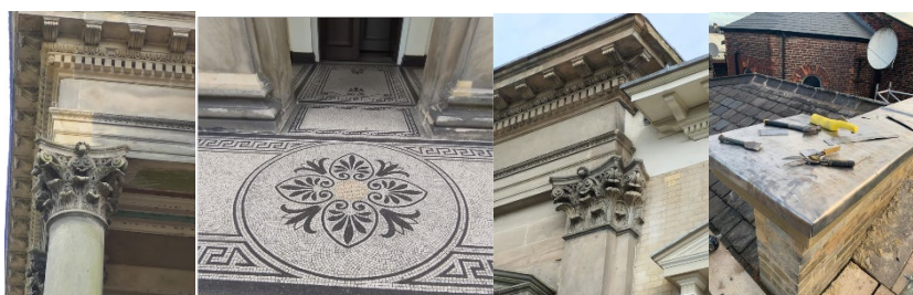
Figure 10. Repairs and Restoration (left to right): Portico 2005-9, Church Roof 2014-5, Presbytery Roof 2022, by author.
