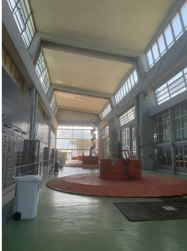
Figure 10. The power plant building (inside). Ph. G. Caudo (August 2023)
