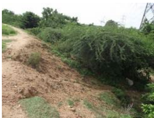
Figure 9. condition of a Tank bund in the study area
