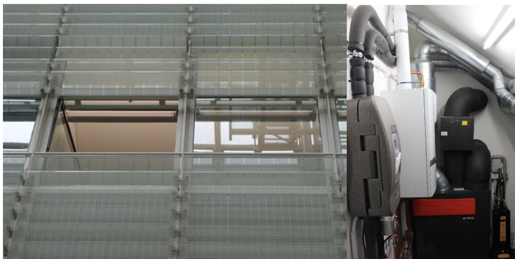
Figure 6. Examples of Enhanced Ventilation Systems – on the left louvre-controlled window ventilation opening and right a heat recovery ventilation system (source: Authors).
