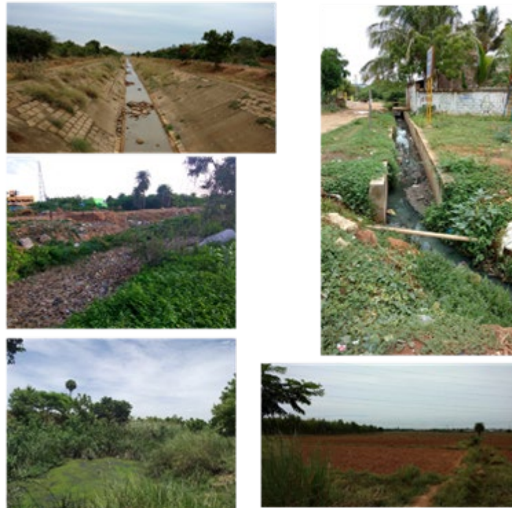
Figure 1. Clockwise from left to right- Damaged channels, Pollution from sewage in the channels, agricultural land converted into vacant plots, Tanks polluted from sewage disposal, channels choked with solid waste
