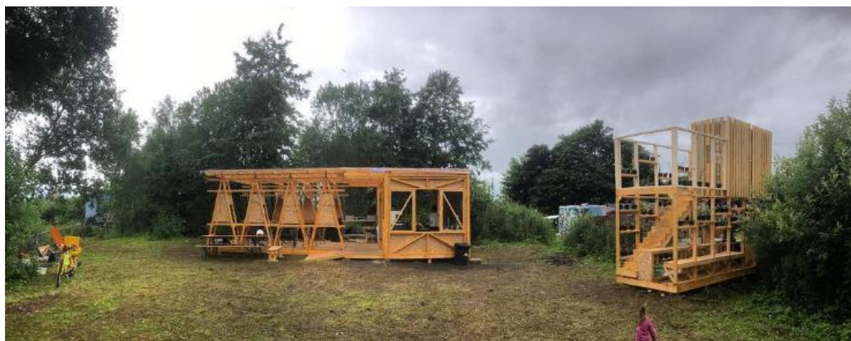
Figure 1: Test Unit, showing main pavilion (left) and ‘The Nettle Inn’ (right) under construction.
